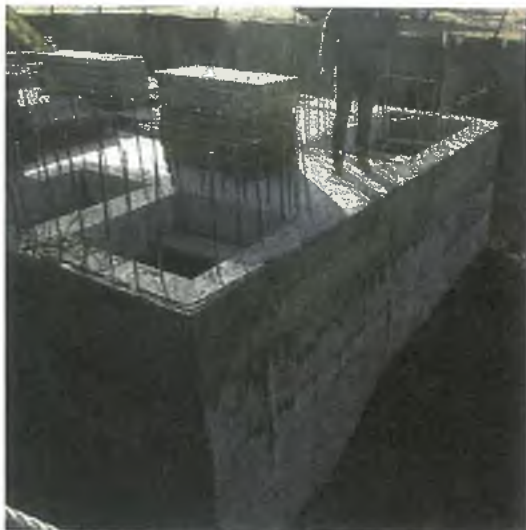
The completed Vortechs® System will be able to meet load bearing requirements for a 747 aircraft.
